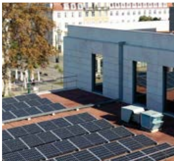
EMSA has 40 photovoltaic panels, covering an area of about 160m 2 as part of the Agency's greening project.
