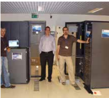
Inside the business continuity data centre in Porto.
