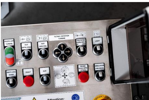
Figure 116: Fixed control panel.
