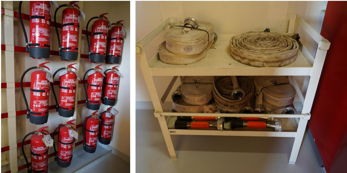
Figure 122: An example of portable fire extinguishers and hoses available onboard a container ship.
