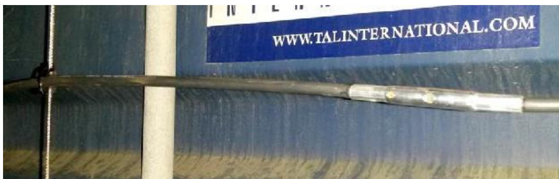
Figure 79: A container wall temperature monitoring sensor installation.
