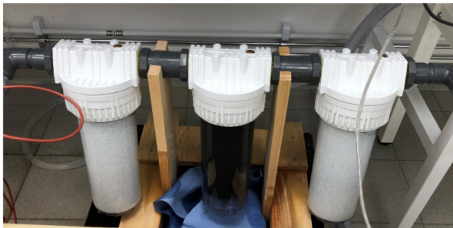
Figure 10 - Filter system used for the holding tank water.
