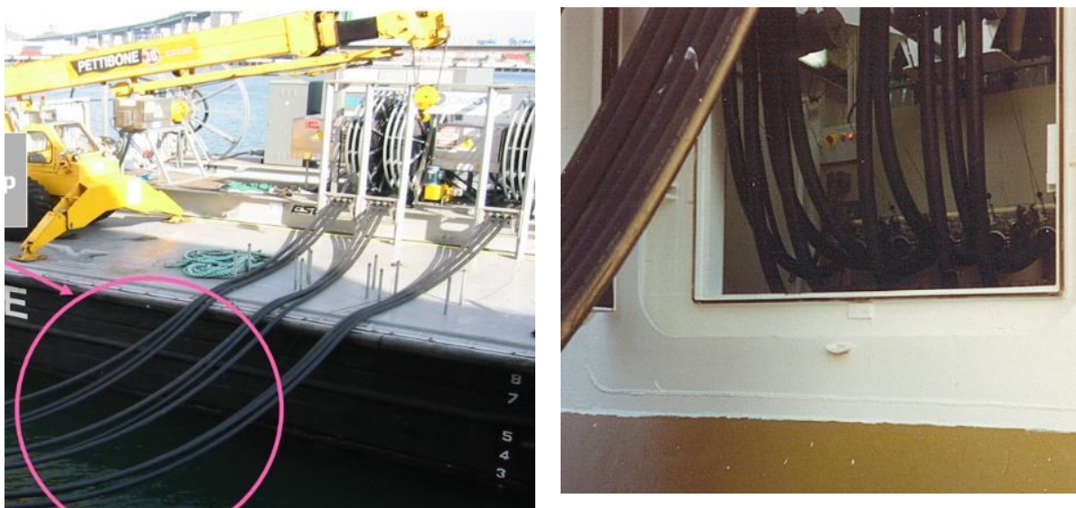
Figure 3.101 (a) and (b) – Multiple electrical cables are involved on low voltage shore connections.
