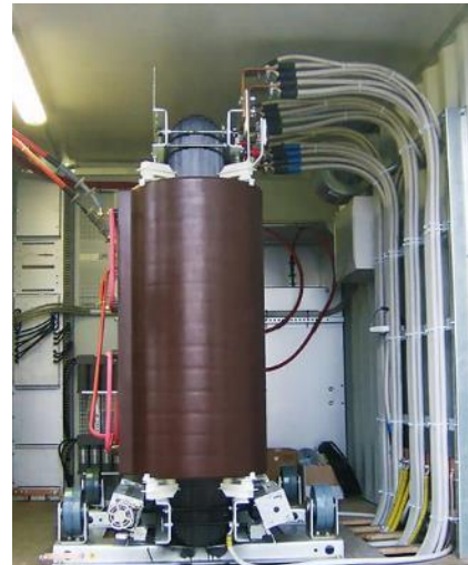
Figure 3.45 – Dry-transformer secondary connections by cable
