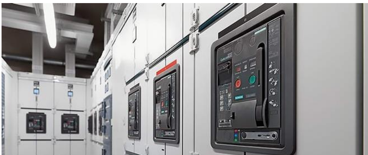
Figure 3.61 – Different panels of a distribution low-voltage switchboard.
