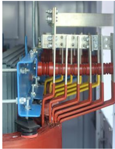
Figure 3.44 – Dry-transformer - secondary winding connections by aluminium busway.
