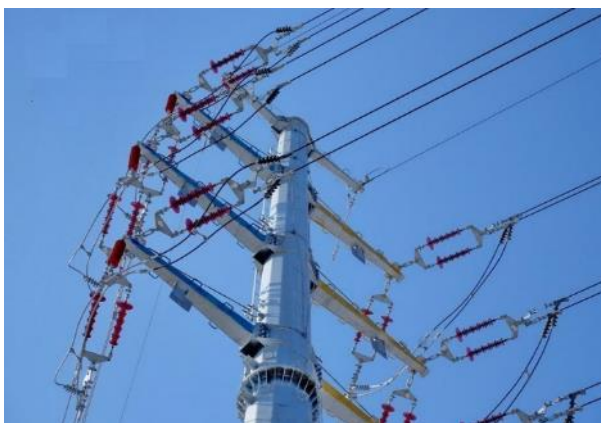
Figure 3.24 – Overhead pole, 33 kV.
