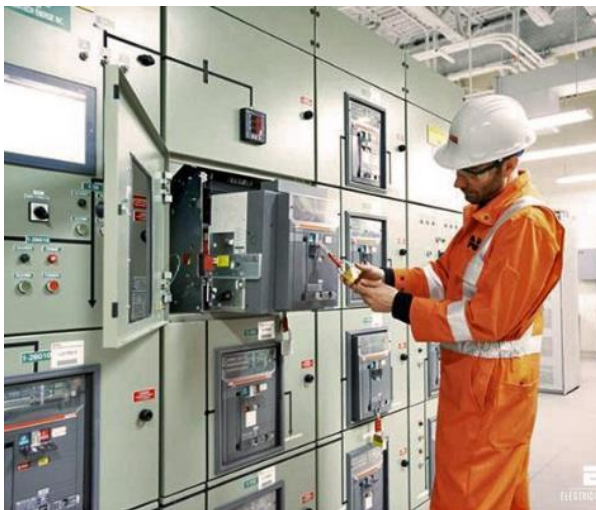
Figure 3.55 – Verification conducted on a circuit-breaker.
