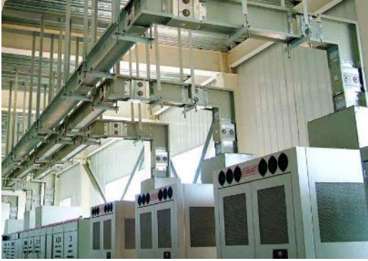
Figure 3.41 – Substation above head busway.
