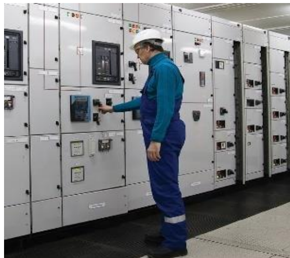
Figure 3.56 – Switchboard operation is done either remotely or locally in the front panels.
