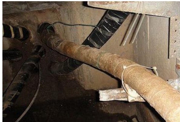
Figure 3.29 – Underground HV cable vaults can be subject to flooding.
