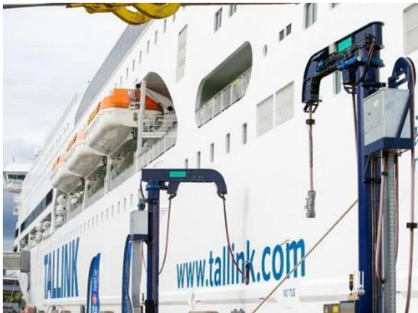
Figure 3.114 – OPS fixed CMS – RO-Pax HVSC supported by crane.
