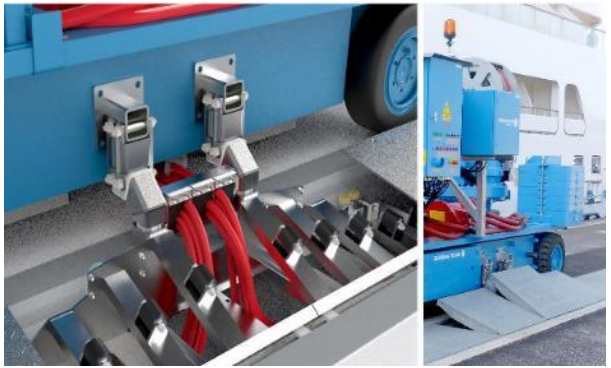
Figure 3.105 – OPS mobile CMS – HV connection of the mobile CMS to a trenching flexible cable tray which runs along the length of the berth.
