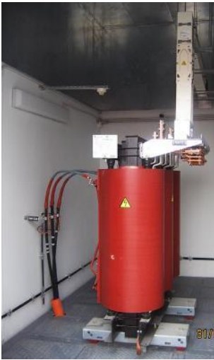
Figure 3.43 – Dry-transformer - secondary winding connections by enclosed busway trunk.
