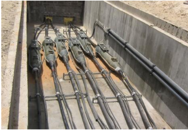
Figure 3.26 – HV cable connections in underground cable vault.
