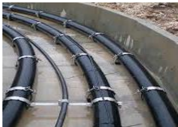
Figure 3.25 – Underground HV cable routed in a special concrete pit near-ground, prior to coverage.
