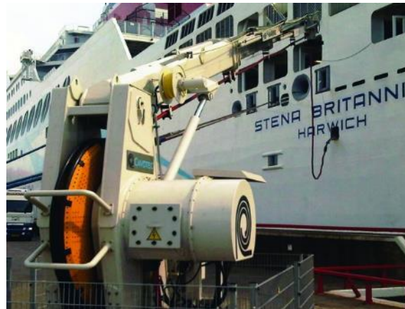
Figure 3.115 – OPS fixed CMS – RO-Pax HVSC supported by hydraulic articulated mechanical arm.
