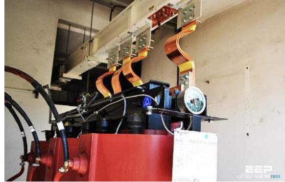
Figure 3.42 – Dry-transformer - secondary winding connections - short bar connection to above head busway.
