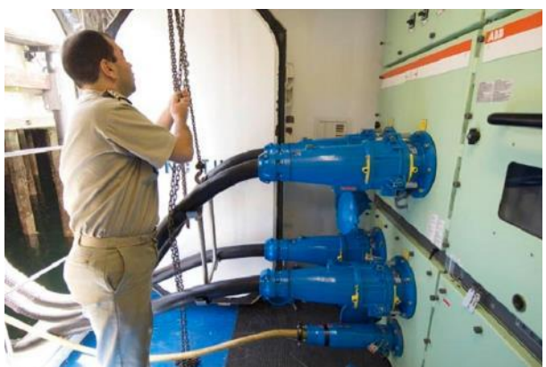
Figure 3.130– Ship side HVSC connector-inlet arrangement onboard a cruise ship including 4 parallel power cables + one neutral.
