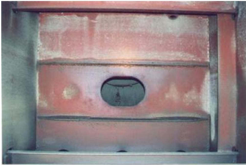
Correct paint application, ballast tank condition after 13 years (a bulk carrier double bottom tank is shown in this example)
