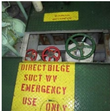
Emergency bilge pump valve
