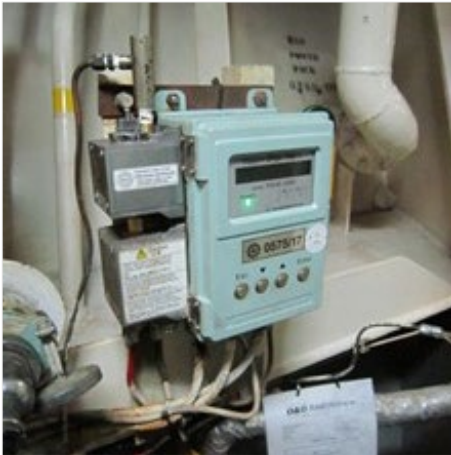
Oily Water Separator
