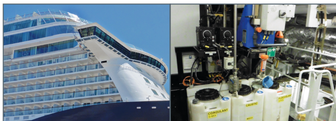
Hybrid scrubber system offers an alternative to lower sulphur fuel
