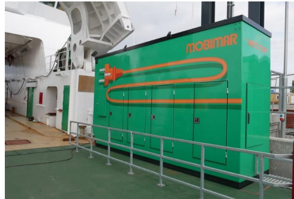
Figure 4.20 – Shore-side Battery Charging – MV Ellen shore-side fast charging transformer.
