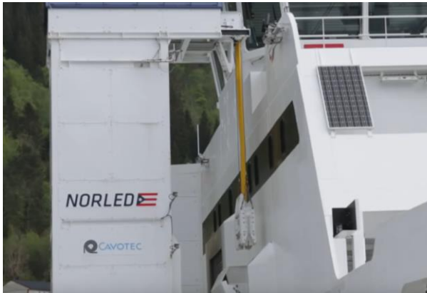
Figure 4.19 - Shore-side Battery Charging – NORLED Ampere – CAVOTEC system with gravity driven charging cables falling into connection.
