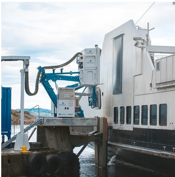
Figure 4.21– Shore-side Battery Charging – induction charging connection.
