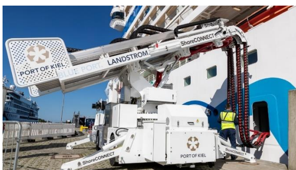
Figure 4.7 - HVSC with mobile CMS – High-voltage shore power supply to cruise ship – high power demand requirement.
