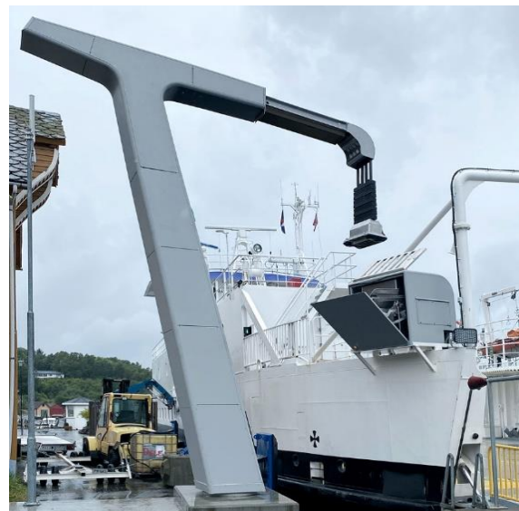
Figure 4.22 - Shore-side Battery Charging – Portico solution for battery charging connection. Several parallel cables grouped, with gravity connection.
