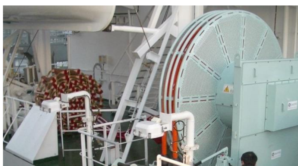
Figure 4.8 - HV Shore Power cable reel onboard a containership.
