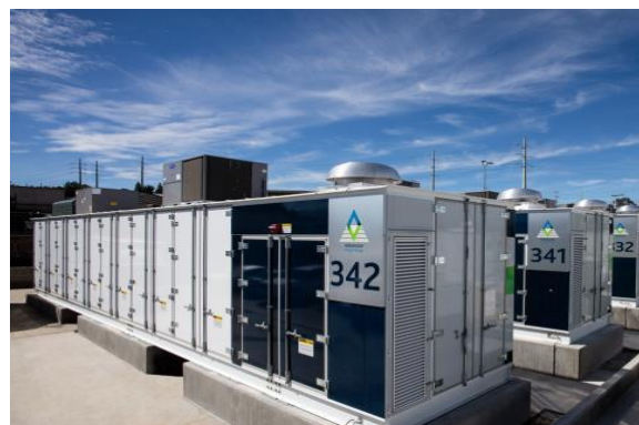
Figure 4.31 - Multi-MW battery bank – to be noted the refrigeration units for the cooling of battery modules.
