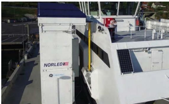
Figure 8.10 – NORLED MV Ampere – Dedicated cable management systems for fast DC battery charging.
