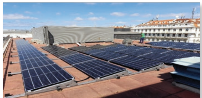
Solar panels on the roof of EMSA's Lisbon headquarters
