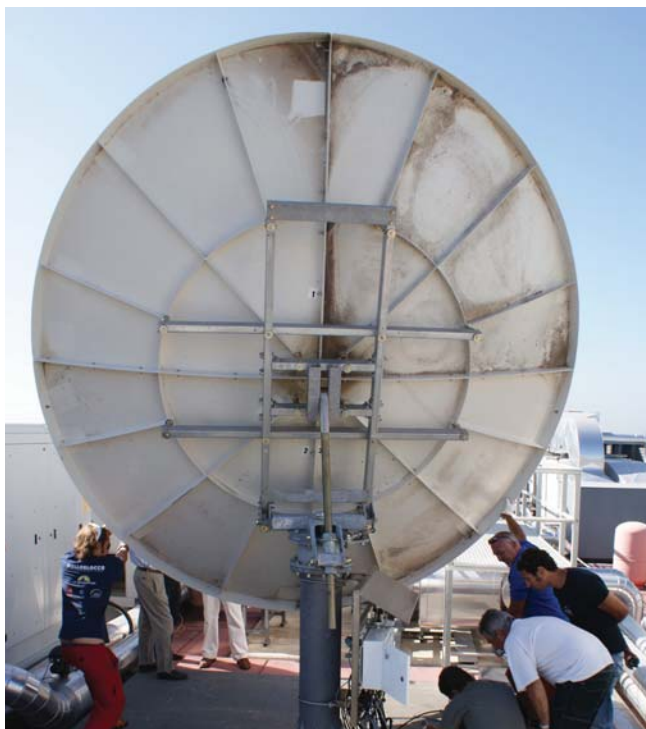
The dish installed on EMSA's roof in 2009 helps ensure secure and fast communication of satellite images.
